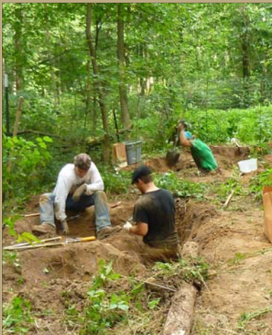
Figure 1. Excavation of roots was completed primarily by hand, though on some larger trees, trenches were dug adjacent to roots with a Bobcat backhoe attachment.
